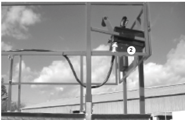
Figure 6.1.2 Control Box Location, Platform Position
