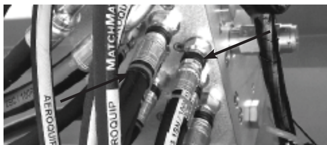
Figure 7.14 - Check Fittings at Valve
