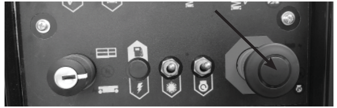
Figure 2.2 - Ground Control Box Emergency Stop Switch
