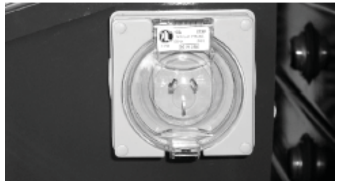
Figure 11.7 - Mains Power Connection For Charger
